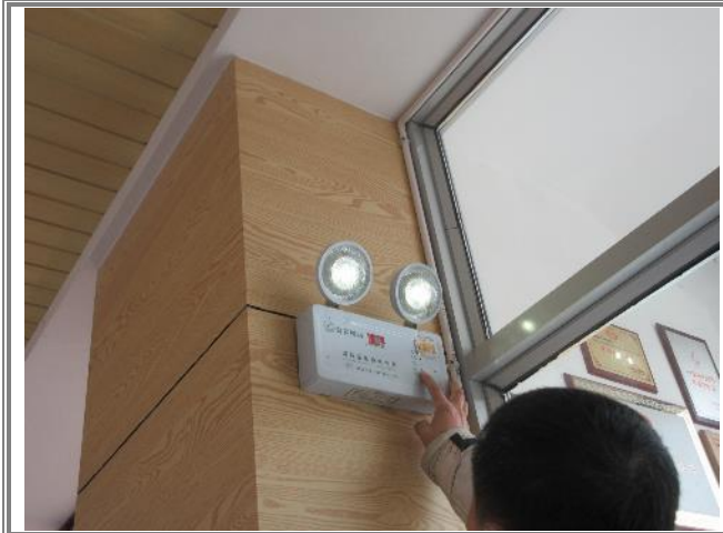
Emergency light testing
