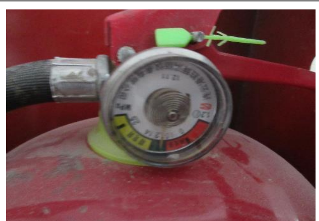
Functional fire extinguisher
